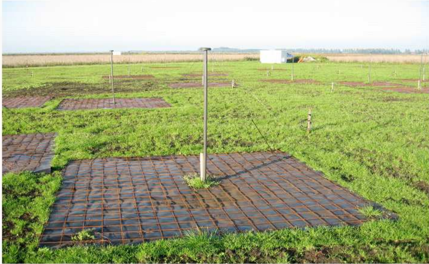
LBA-antenna (4 wires, 2 pol) + ground plane
